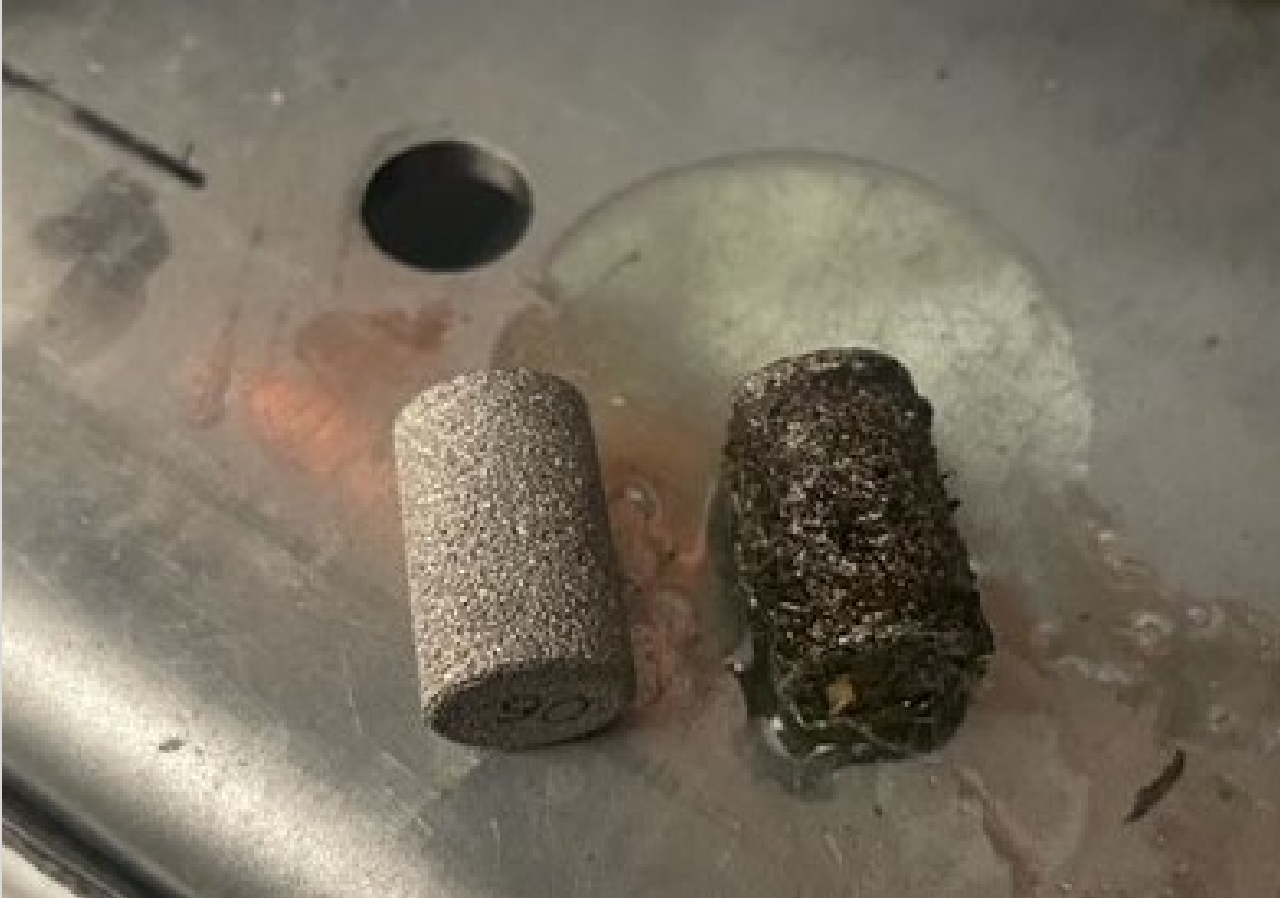
Low Oil Reservoir Alarm
